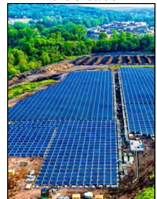
Solar Installation At The Transfer Station
